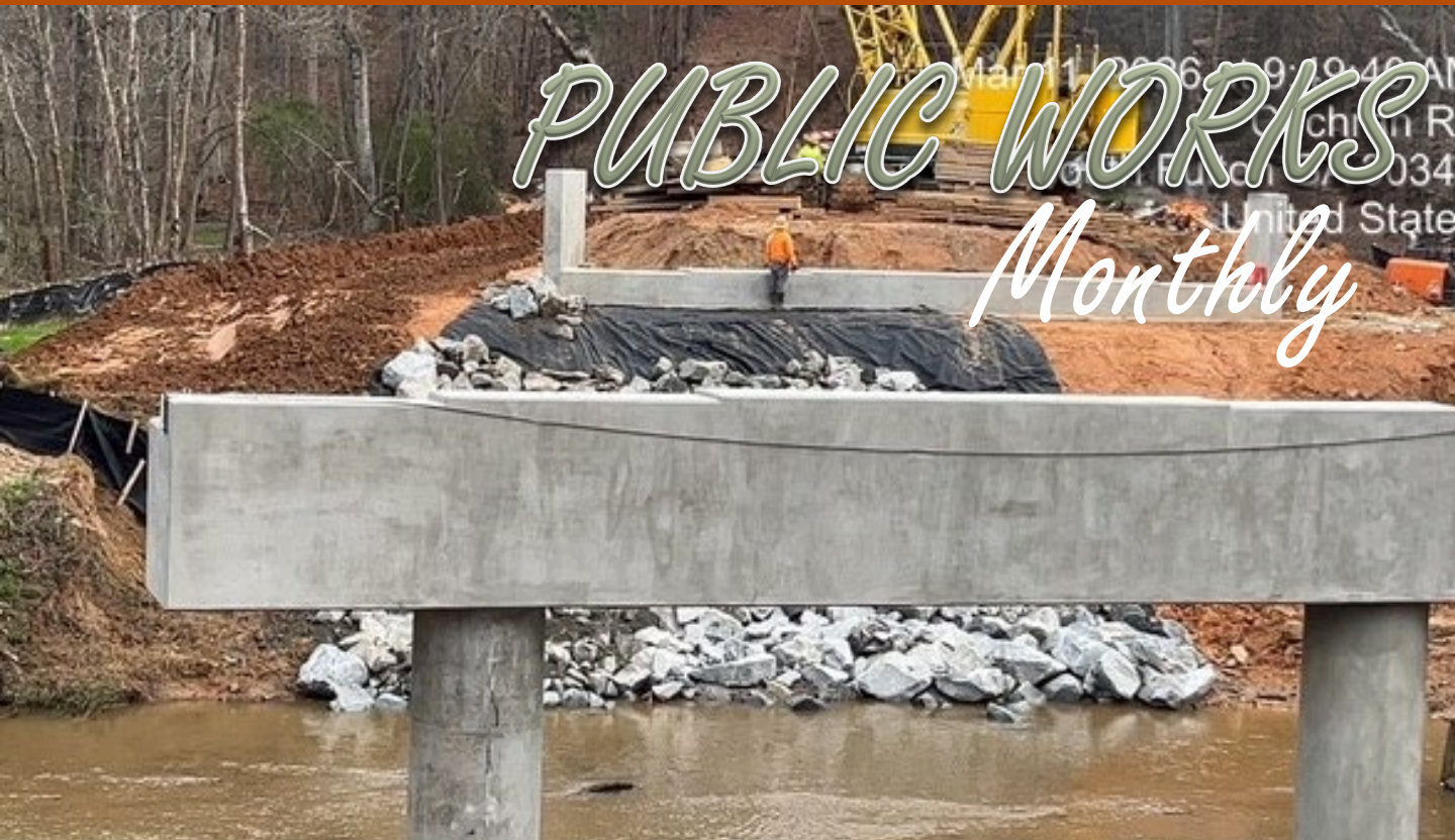
Cochran Rd Road over Camp Creek Bride Replacement: Bridge bents & rip rap installed on slope
