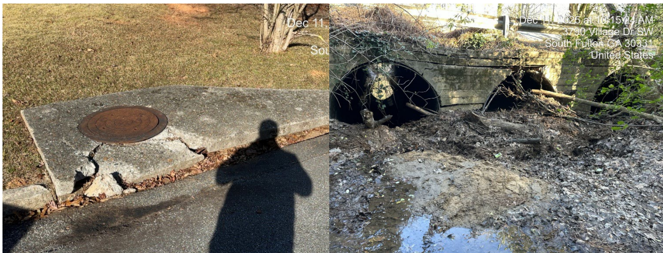
(from left to right) storm Inlets 1. damaged by vehicle traffic 2. Triple 72-inch culvert with failing headwall and debris
