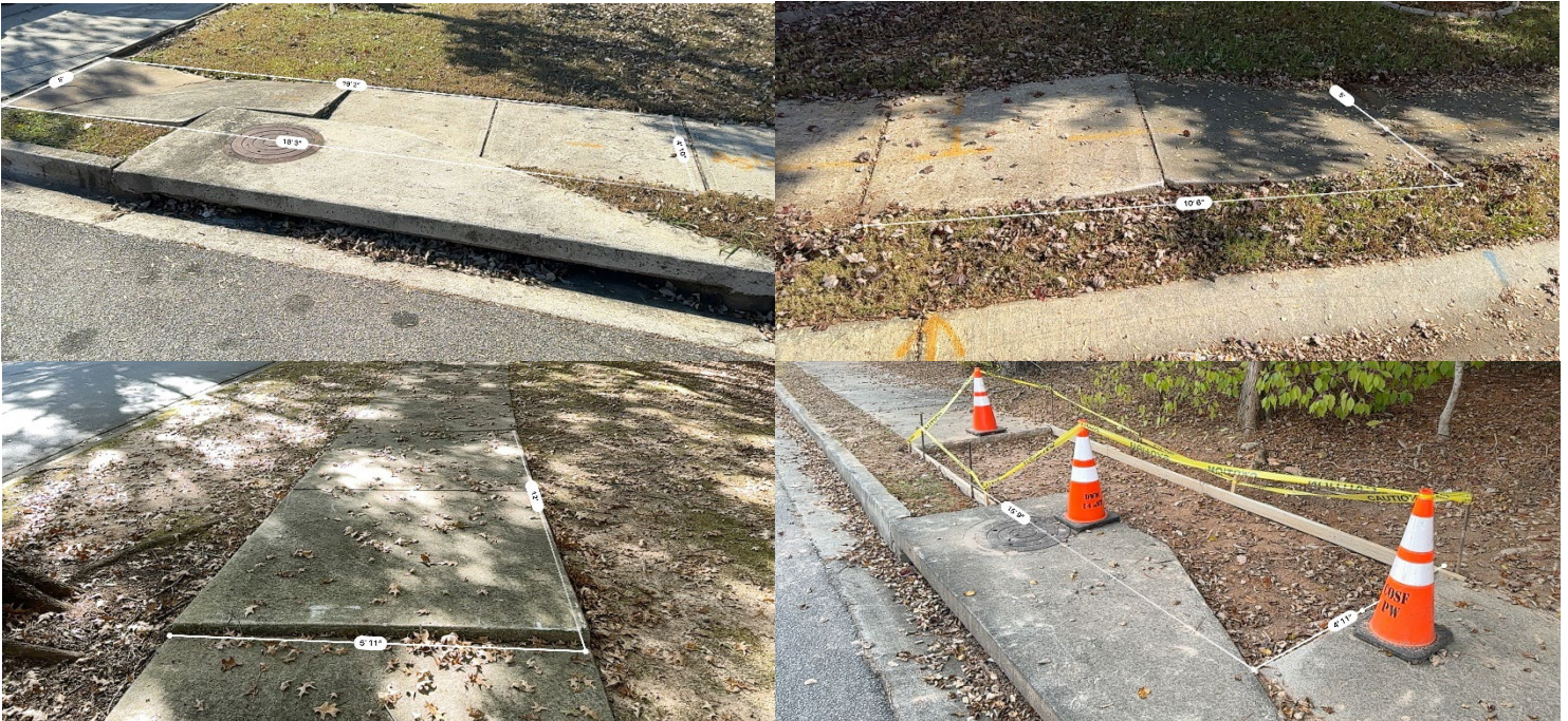
Pending Sidewalk repairs (District 4)
