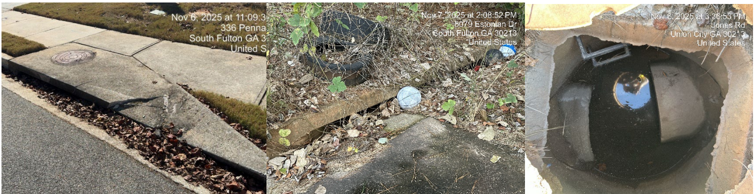
(from left to right) District 4 storm Inlets 1. damaged by vehicle traffic 2. blocked with debris 3. Standing water due to blockage
