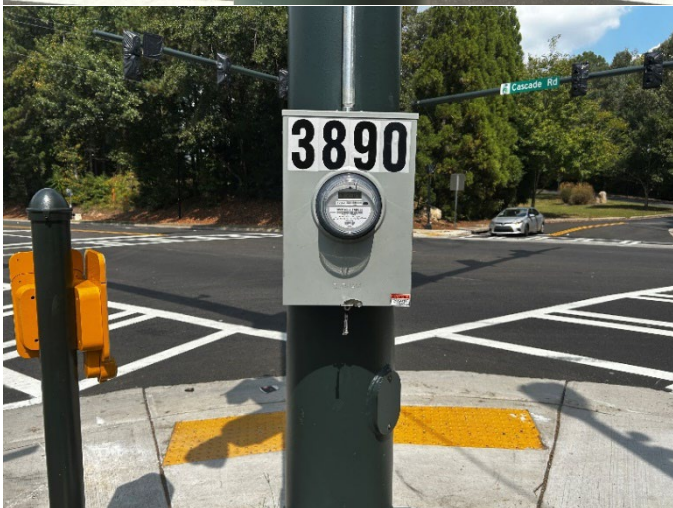
Traffic Meter Install
