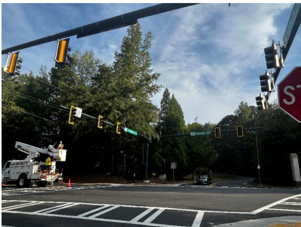
Intersection Traffic Devices Activated
