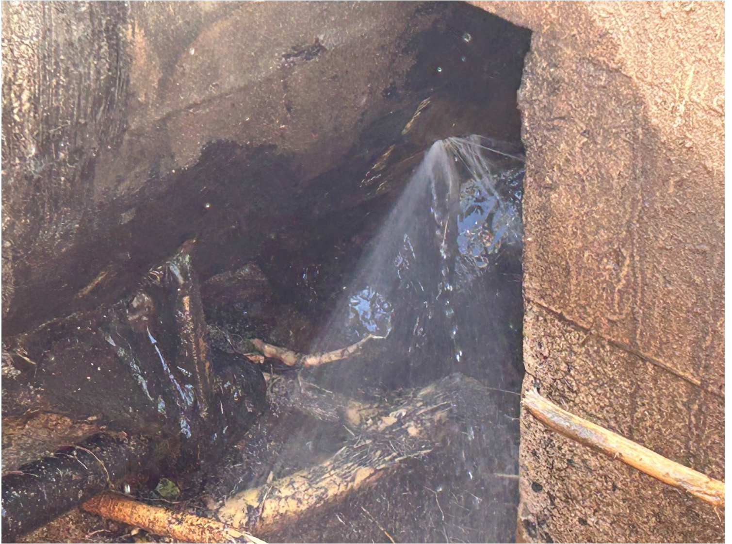
30 in. Water main leak
