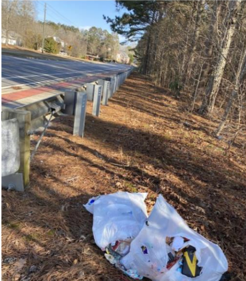
Illegal dumping located at big bridge on Bethsaida Rd - December 2020
