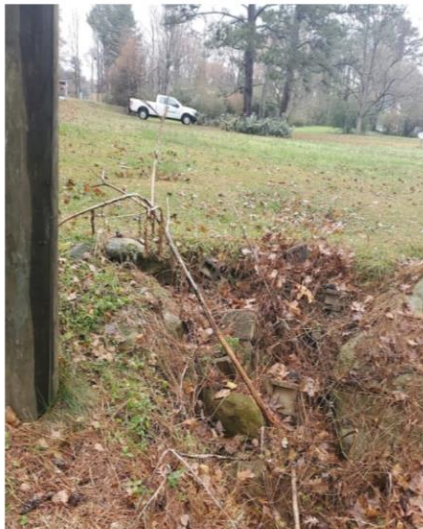
Blocked drainage pipe outlet located off Old Bill Cook December 2020
