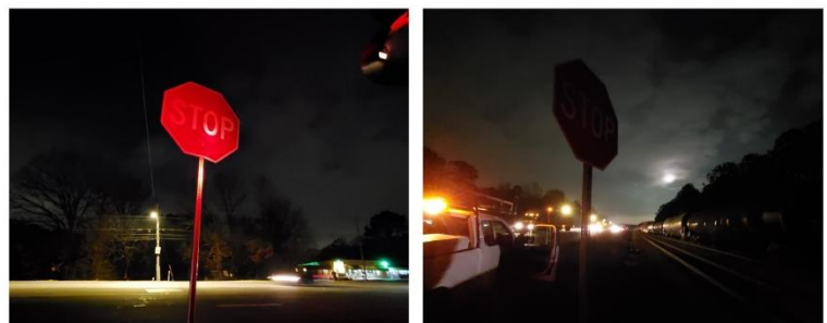
Damaged sign repair along Roosevelt Highway December 2020
