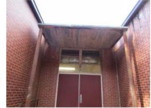
Corroded Steel Canopy
