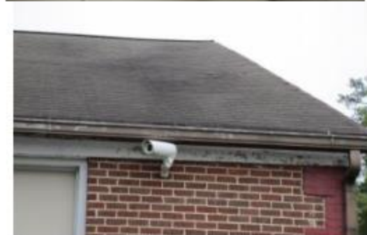
Deteriorated and Lifting Shingle Roof
