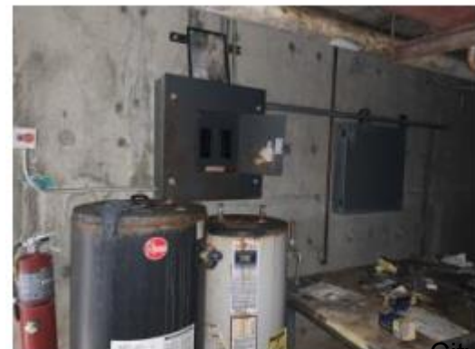
Water Heater and Panels
