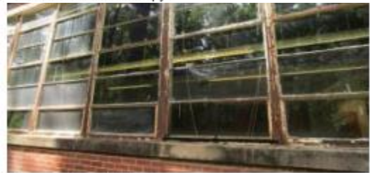
Corroded Steel Windows
