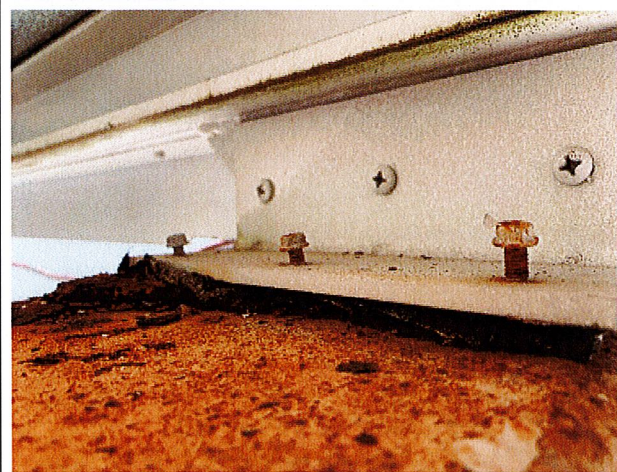
5. Corrosion and withdrawing structural fasteners.
