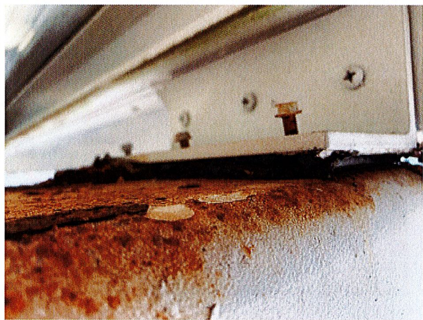
4. Corrosion and withdrawing structural fasteners.
