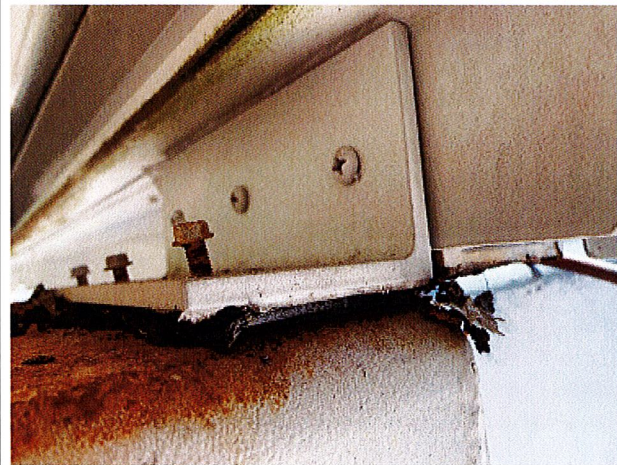
3. Corrosion and withdrawing structural fasteners.
