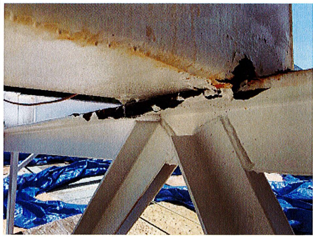
2. Severe corrosion at connection between truss top chord and hollow structural section (HSS) purlin.
