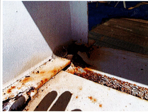
1. Severe corrosion at connection between top side of truss top chord and bottom flange of wide-flange purlin.
