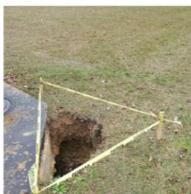
Sinkhole located at Sundridge Dr March 2021
