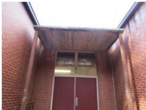
Corroded Steel Canopy
