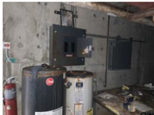
Water Heater and Panels
