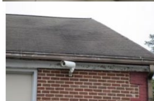
Deteriorated and Lifting Shingle Roof
