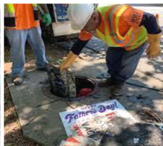
Signs Removed from Storm System at Cascade and Utoy
