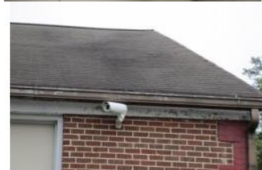
Deteriorated and Lifting Shingle Roof
