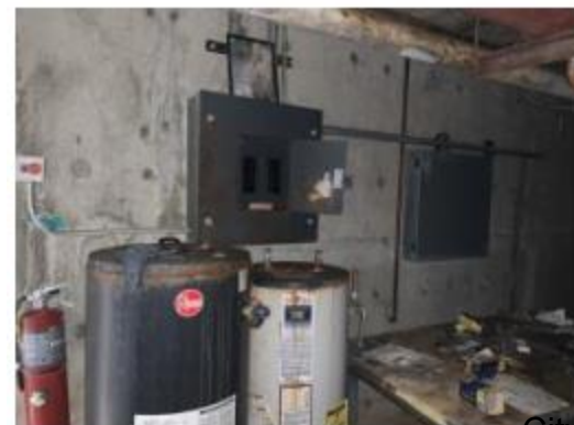
Water Heater and Panels
