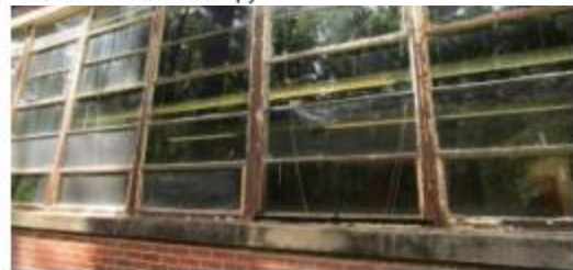
Corroded Steel Windows
