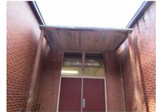
Corroded Steel Canopy
