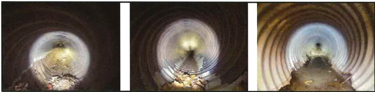
Storm Pipe Minor Corrosion
