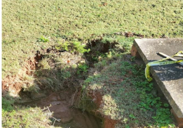
Sink Holes Forming Due to Failure in Pipe & Grouting Around Junction Boxes Melanie Lane – October 2020
