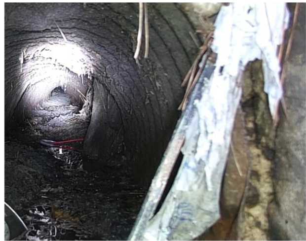
Flood Water Inside A Storm Water Pipe Cedar Wood Court October 2020
