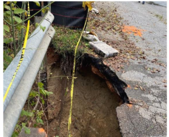
Stacks Rd Bridge approach washed out during Tropical Storm Sally October 2020
