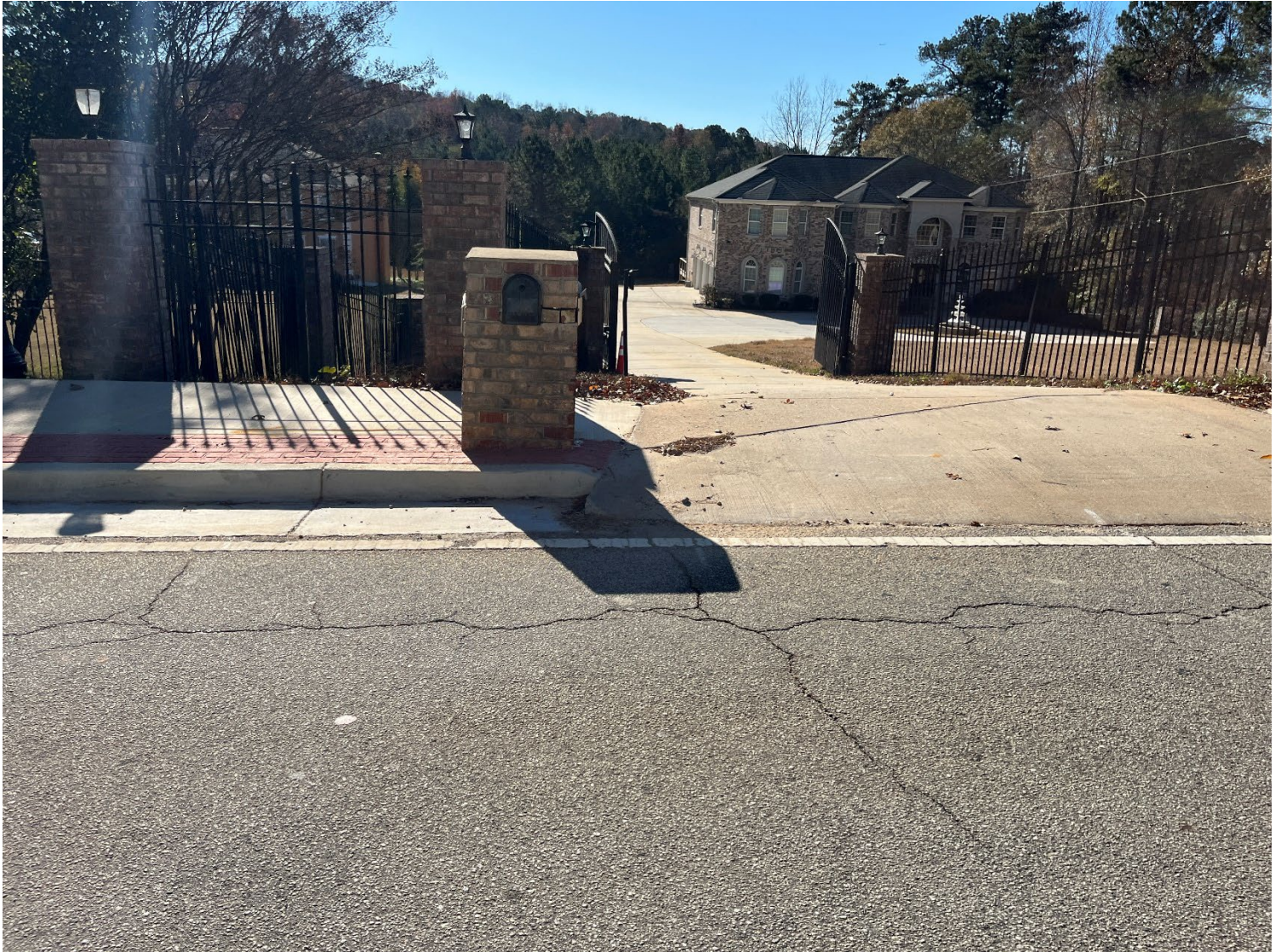
Driveway and Valley Gutter needs to be reconstructed once mailbox is rebuilt
